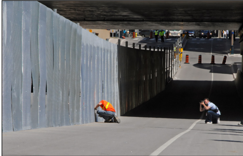
Figure 6: June 8 - Fence under construction on Lower Simcoe St. near Bremner Blvd. (Photo by Tomasz Bugajski)
