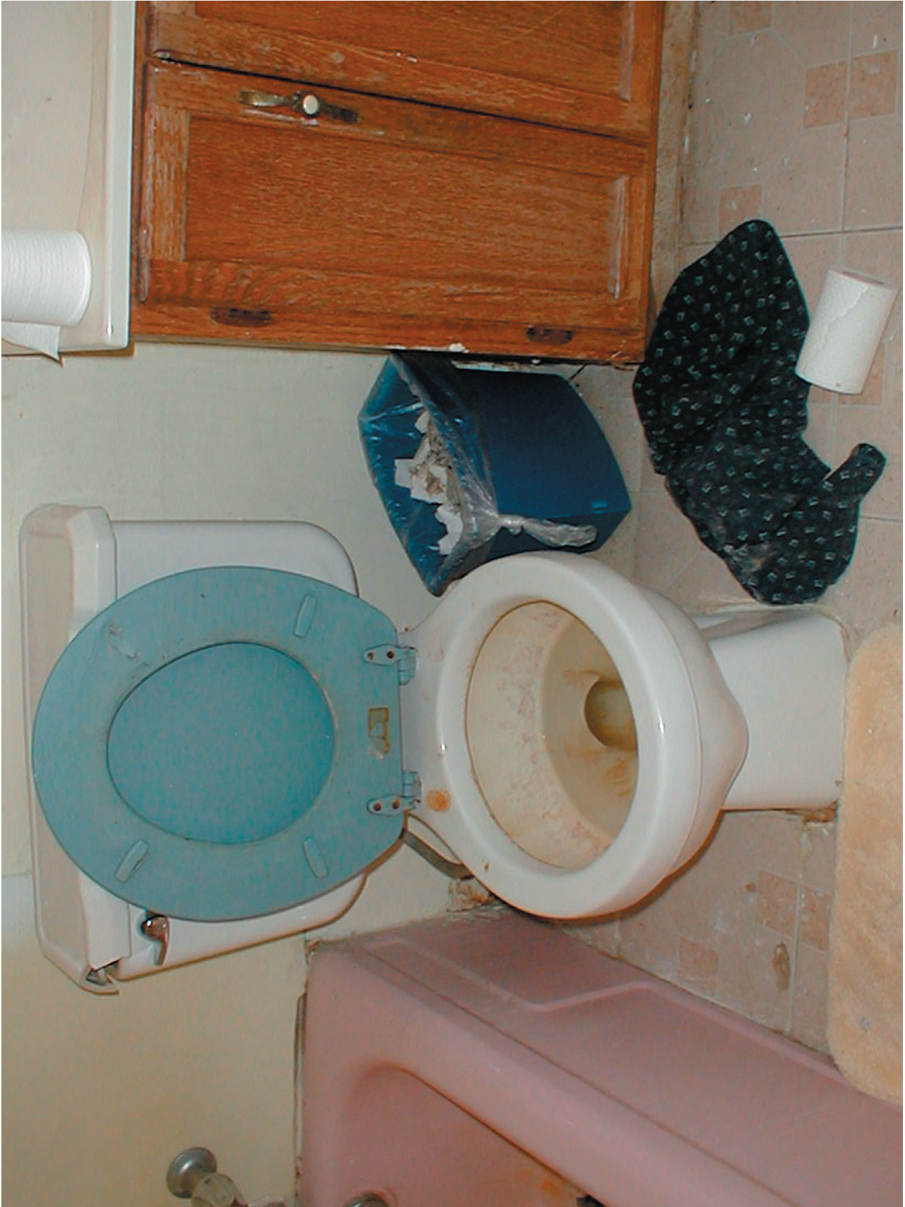
Bathroom at a residential treatment center that cares for both male and female foster children. This facility receives a daily rate from DPRS for each foster child ranging from $80 to $115.
