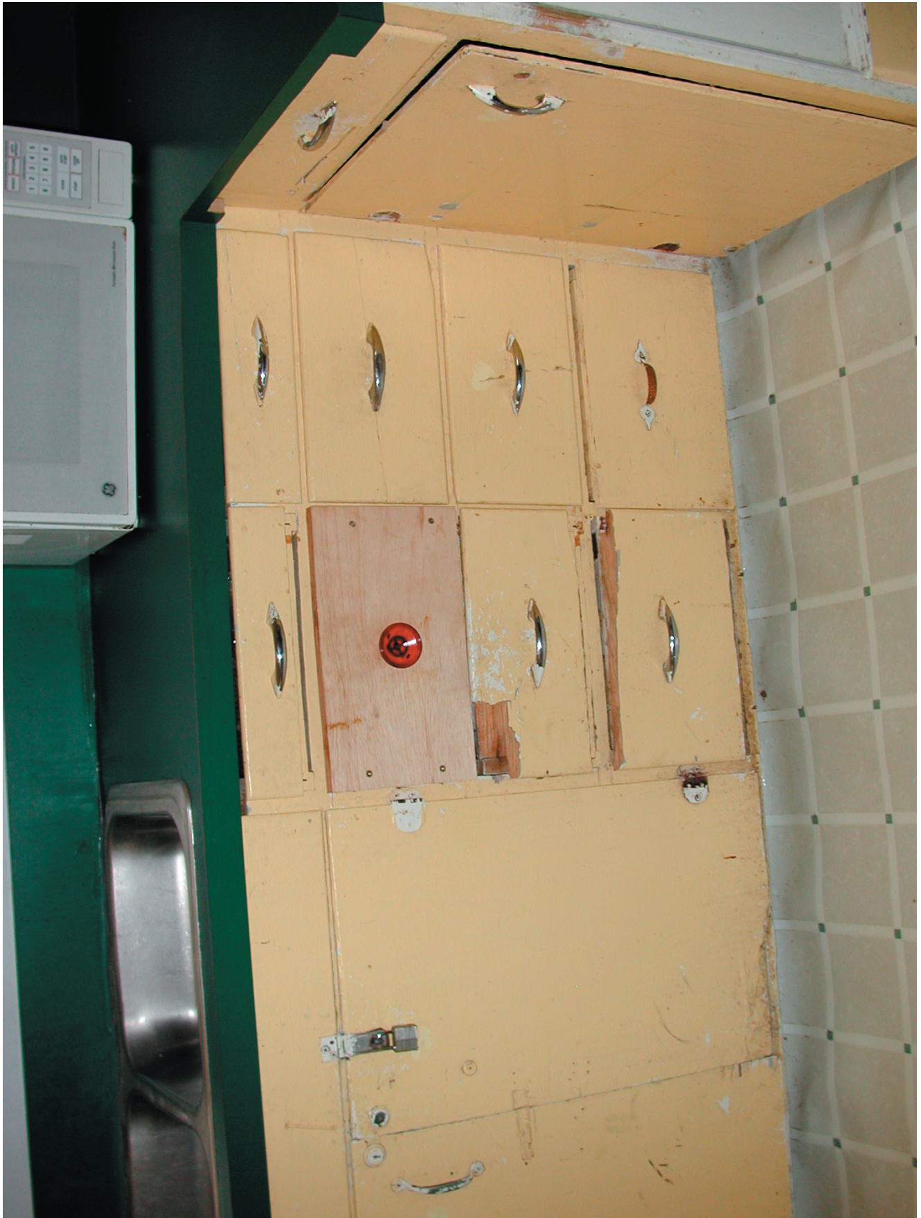
Kitchen at a residential treatment center that serves foster children. This facility receives a daily rate from DPRS for each foster child ranging from $80 to $115. This facility has been found to be deficient in meeting standards for food preparation.
